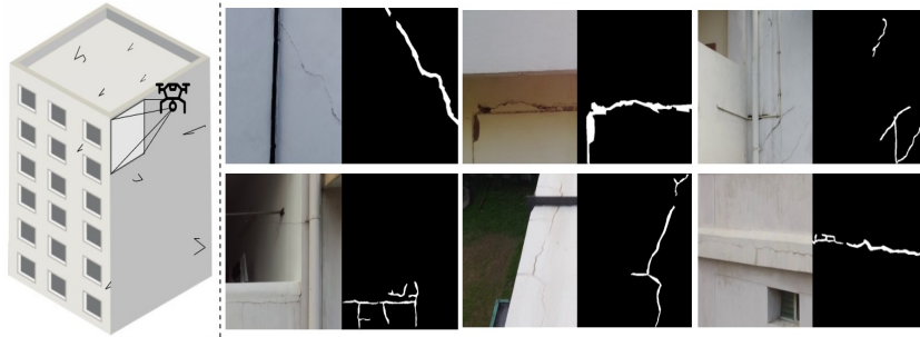
Fig. 1. BuildCrack dataset was captured by imaging building facades using a drone-mounted camera from different angles and distances. BuildCrack has images with low contrast, occlusions, and shadows, which challenge the model’s robustness. Sample images from our building crack dataset are shown. This dataset will be made public.
