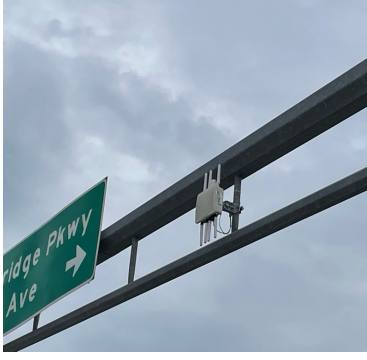
(a) RSU installed at the intersection.
