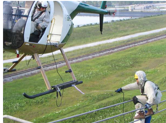
Fig. 1: An operator climbing back to the helicopter after performing maintenance on the conductors.
