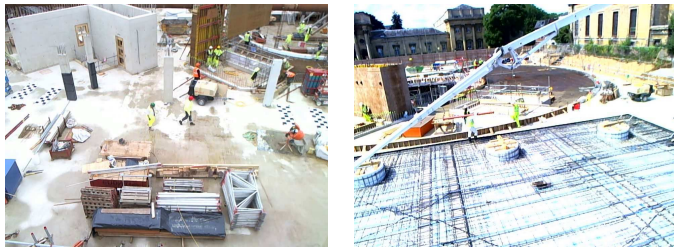
Fig. 2: We have conducted tracking experiments in a construction site setting: (a) the construction site on day 1, (b) the construction site on day 36. The site changes rapidly from day to day, precluding the use of positioning systems which rely on stable, long-term maps.
