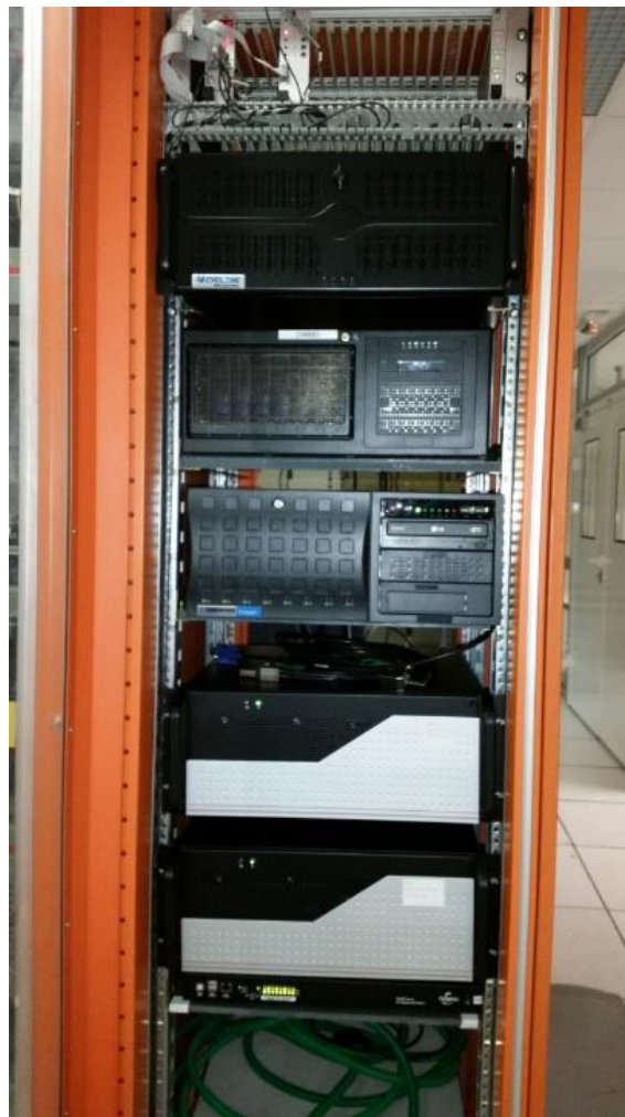
Figure 4 : WMS electronic rack
