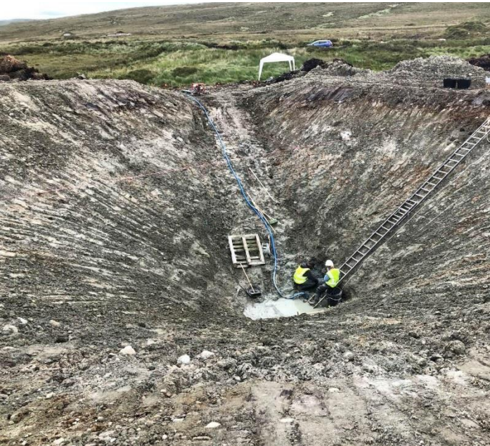
Figure A2. Excavation in 2019 to depth of 5.7 m and showing access ramp, submersible water pump and hose, and exit ladder. Examining the bottom and recovering rock fragments had to be done by feel at this stage.
