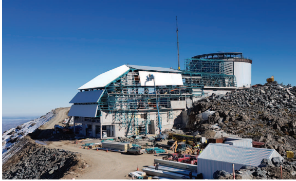
Figure 1. Construction progress of LSST at Cerro Pachon, Chile as of 14 July 2017; for current progress see https://gallery.lsst.org/bp/#/
