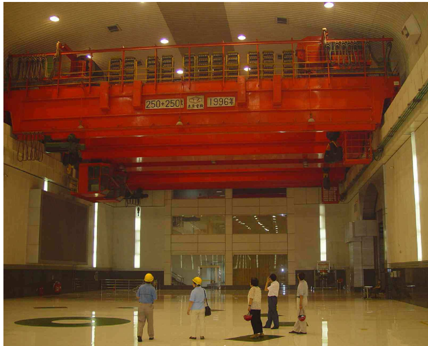
Fig. 4.12. A photo of a bridge style crane, the crane rail is fixed to the wall of the experimental hall.
