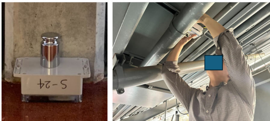
Figure 9: Sensor installation in Stadium 1. The vibration device is shown on the left, and the sensor deployment demonstration is shown on the right. Sensors are strategically placed beneath the cement in seating areas to enhance connectivity.
