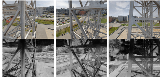
Fig. 1. RGB (top) and thermal (bottom) renderings from our reconstruction of a large crane structure, based on images collected by a Skydio drone. Thermal imaging with 3D reconstruction can be used for building and infrastructure inspection, among many other applications ranging from agriculture to search and rescue.
