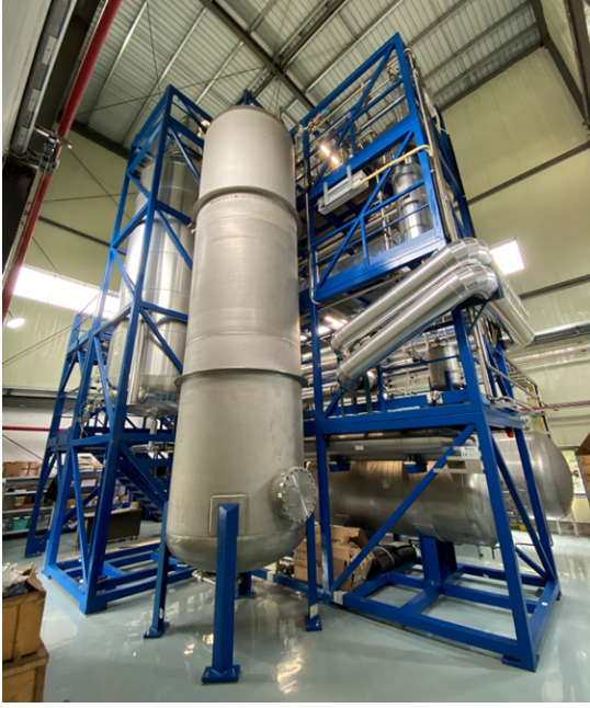
Figure 3: Distillation plant installed in the Over Ground LS building at JUNO site.
