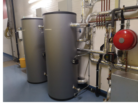
(b) Two 500L water tanks.
