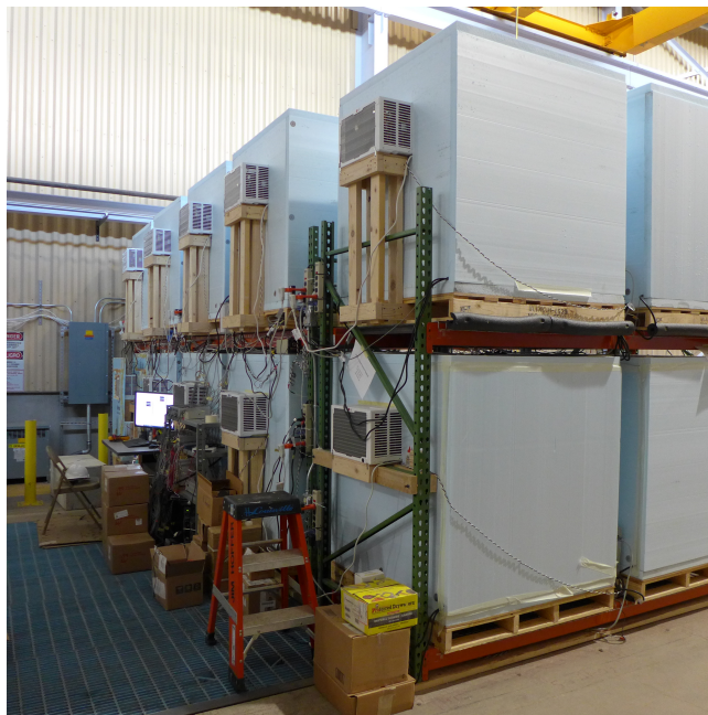
Figure 2: The 20 units are stacked in pallet racks, minimizing cable lengths and overall footprint. In spite of their close proximity to one another, the ACs are not found to synchronize.
