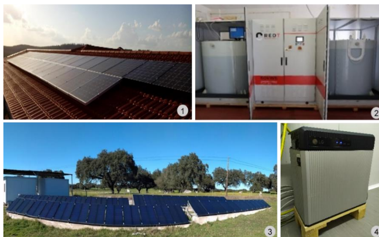
Figure 2. PV systems and BESSs in the Renewable Energies Chair of the University of Évora microgrid: 1) 6.7 kWp crystalline PV installation; 2) 5 kW/60 kWh VRFB, from redT [32]; 3) 3.2 kWp amorphous BAPV system; 4) 5.0 kW/9.8 kWh LIB RESU10 battery pack, from LG [33].
