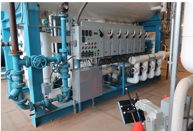
Fig. 37. NIST central utility plant (CUP). Channel sounding experiments in this location were conducted to characterize dense multipath scattering environments. Photo credit: NIST.
