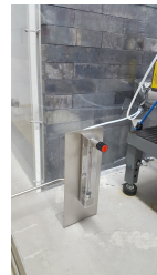
Figure 24: ATEKO-Air Rotameter with valve to measure and regulate air flow rate.
