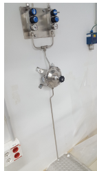
Figure 23: ATEKO-Air main line in Hall C.
