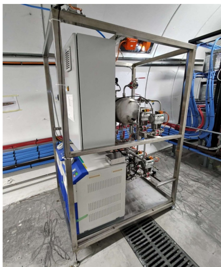
Figure 16: Photograph of the cooling system.
