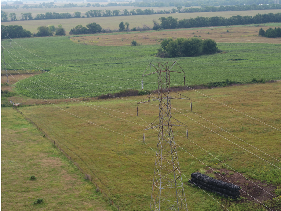
Fig. 2. An example of a power line image.
