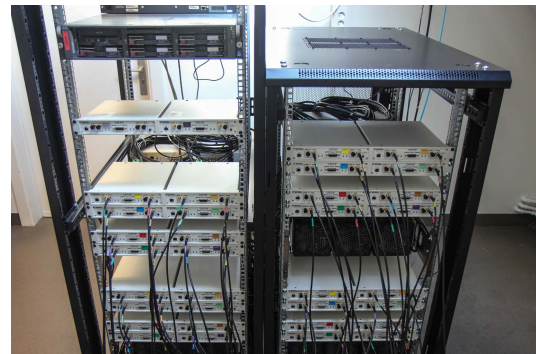
Fig. 8. Measurement setup: power gain variations across the array were calculated from LTE-like uplink data symbols in the KUL massive MIMO test bed. 32 antennas were used in this measurement.
