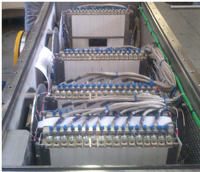
Figure 11. The first five CHANTI stations assembled in their vacuum vessel.
